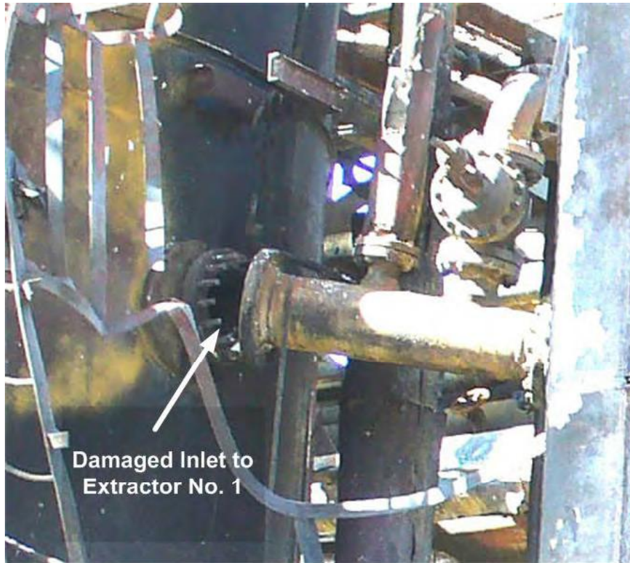
Figure 8. Damaged 10" propane inlet on Extractor No. 1
