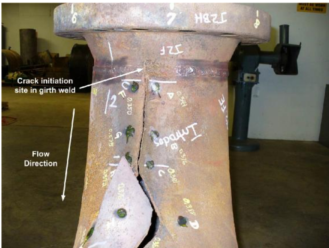
Figure C- 1. Fractured inlet elbow
