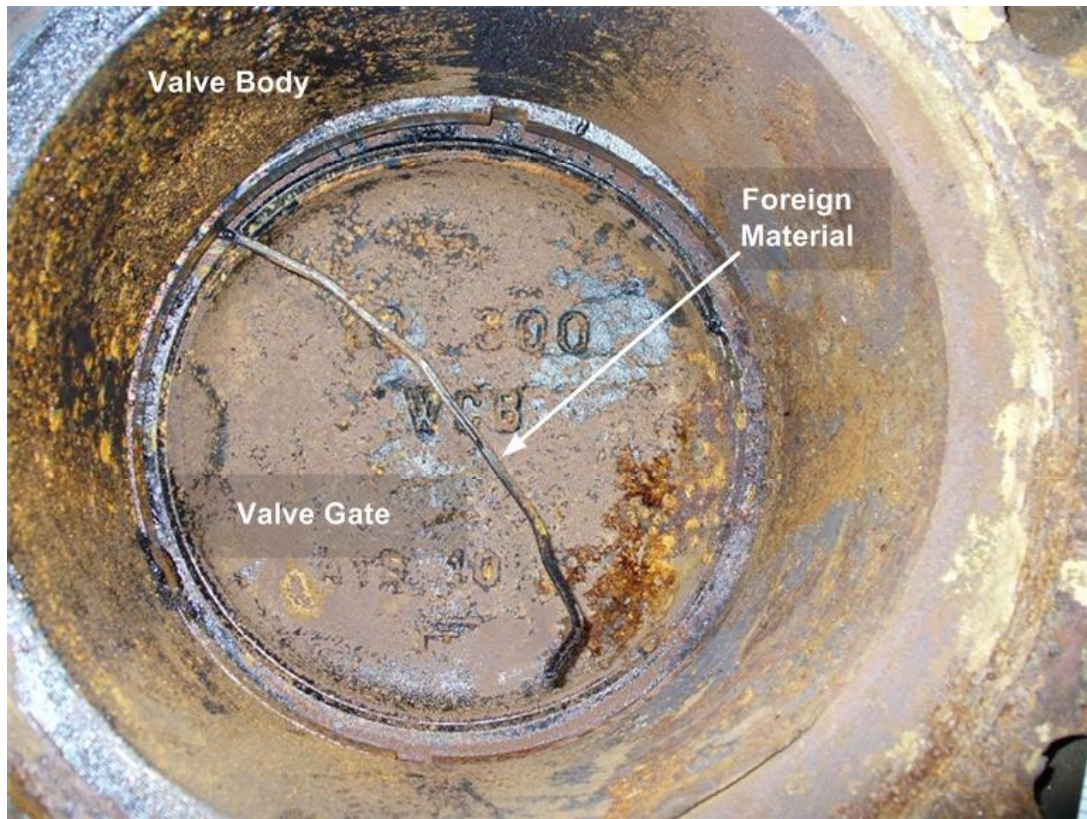
Figure 7. Downstream view of propane mix control station inlet block valve
