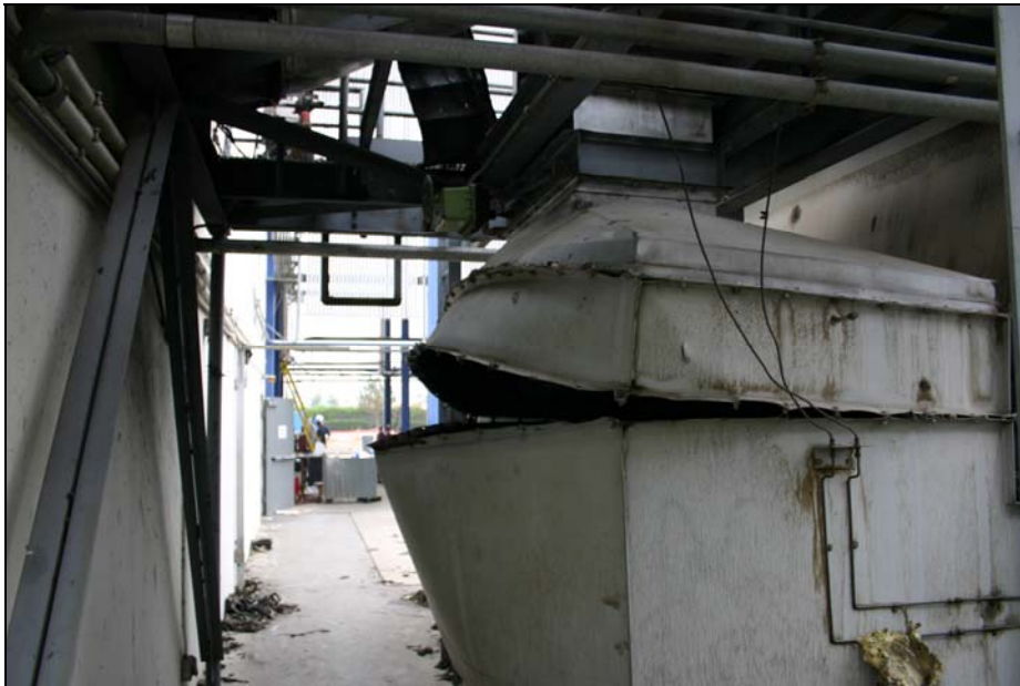
Figure 10 Oxidizer Manifold Damage
