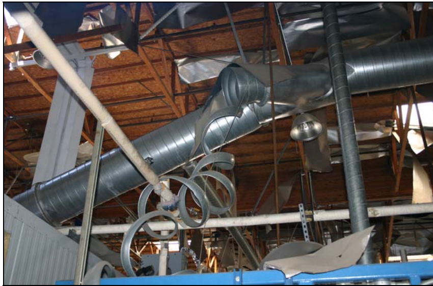
Figure 11 Damage to Ventilation Ducting
