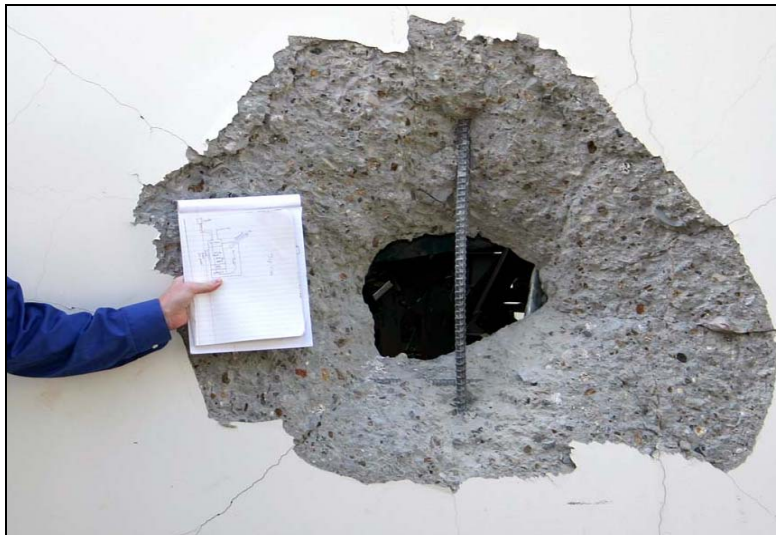
Figure 12 Building Damage from Chamber Door
