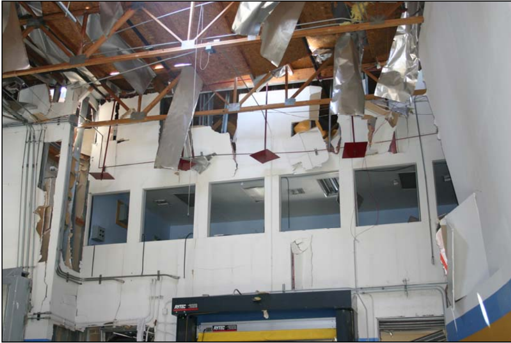
Figure 9 Blown Out Control Room Windows
