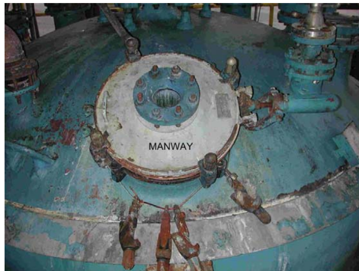
Figure 6. The 18-inch reactor manway.
