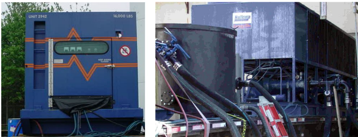
Figure 4. Portable cooling system used to cool the reactor. Generator (left), and chiller (right).
