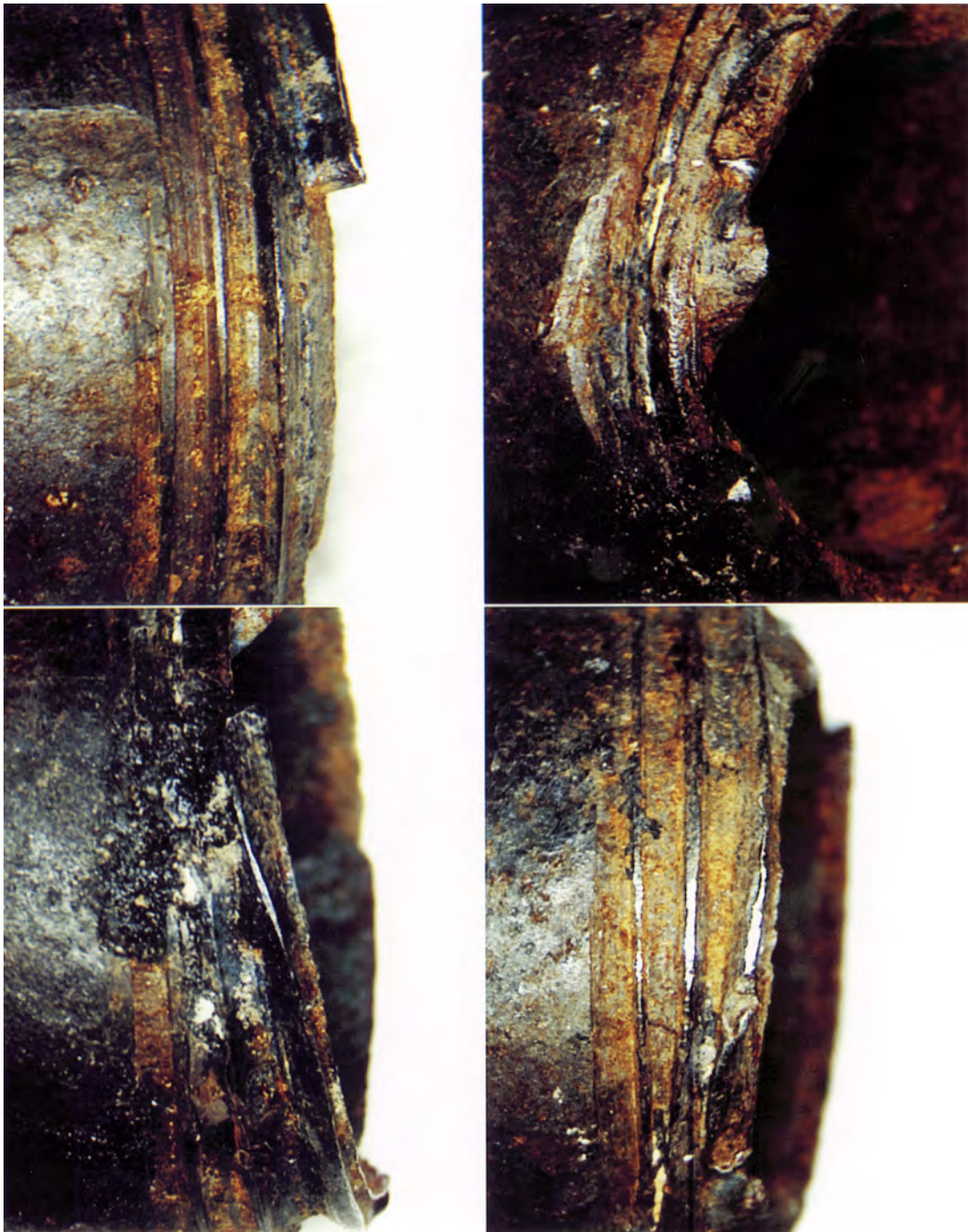
Figure 39 90° rotational view of the condition of the pipe threads on the one inch pipe (A1). MAGNIFICATION: 5X
