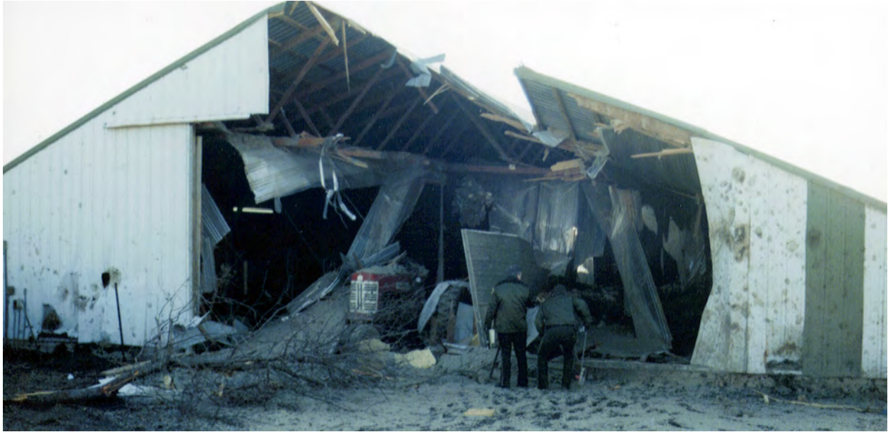
Figure 11. Damage to West End of Turkey Barn (1f)
