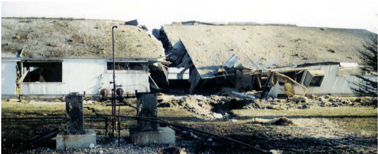
Figure 12. Damage to Turkey Barn (1g) Caused by Impact of Large Tank Fragment
