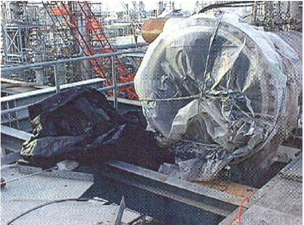
Figure 2. Clear Plastic Sheet Covering One Of The Pipe Openings
