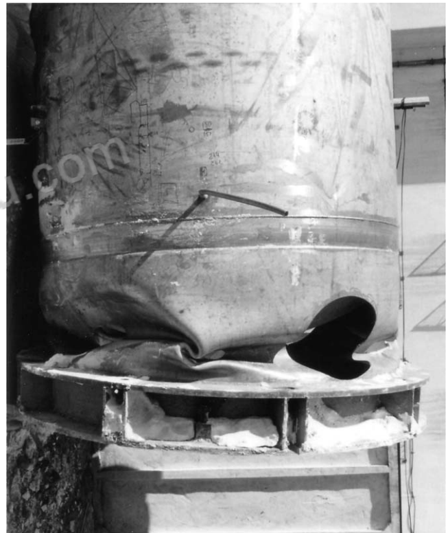
Fig. 12. HP column, buckled skirt.
